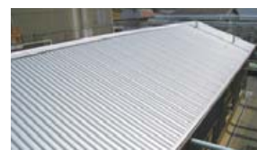
A roof with thermal insulation improved by making the slate roof into a double-layered structure
