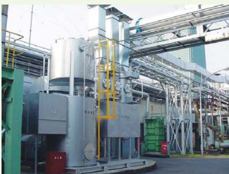
Exhaust gas treatment facilities
