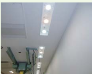
Energy conservation through a switchover to LED lighting equipment (Amagasaki Plant)
