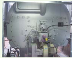
A boiler that has been converted for gas usage (Shizuoka Plant)
