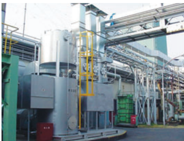
Exhaust gas treatment facilities
