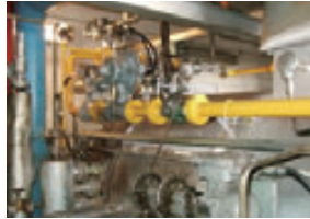
Pipes for natural gas transport at a boiler that has been converted for gas usage (Shizuoka Plant)
