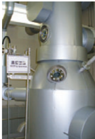
Distillation recovery equipment for waste isopropyl alcohol
