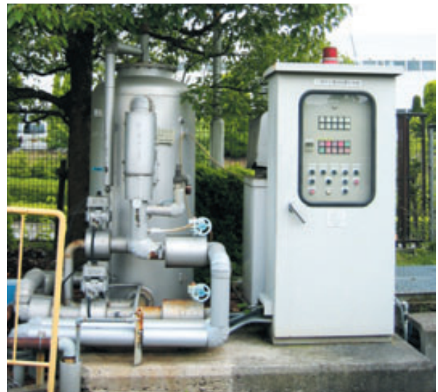
Rainwater treatment equipment (Nara Plant)
