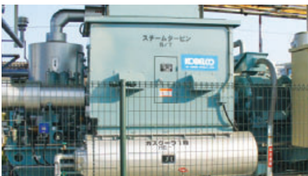
Steam turbine compressor (Shizuoka Plant)
