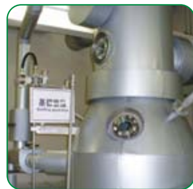
Distillation recovery equipment for waste isopropyl alcohol
