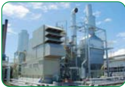
Cogeneration system (Shizuoka Plant)
