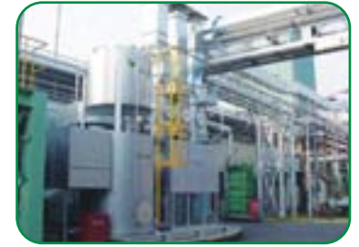
Exhaust gas treatment facilities
