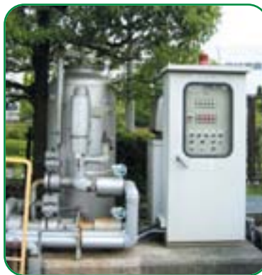
Rainwater treatment equipment (Nara Plant)
