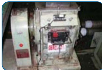
Safety countermeasures for pulverizer (Amagasaki Plant)
