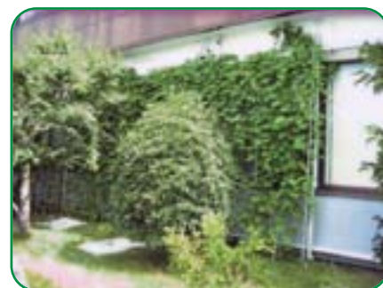
Energy conservation via greenification (Nara Plant)
