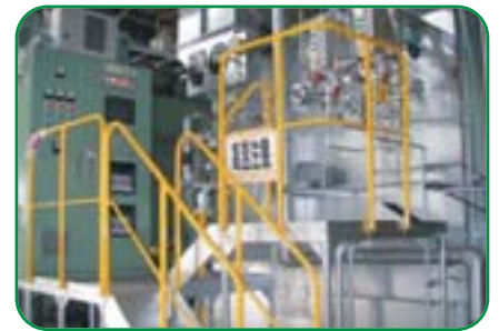
Boiler converted to utility gas (Amagasaki Plant)
