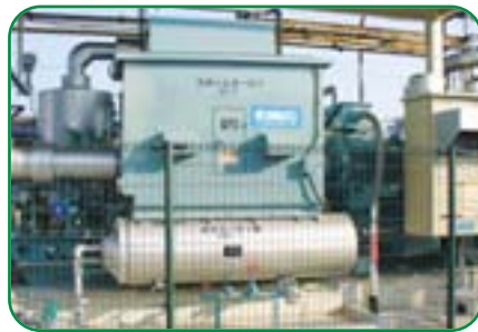
Steam turbine compressor (Shizuoka Plant)
