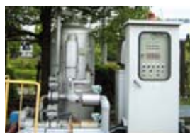
Rainwater treatment equipment (Nara Plant)
