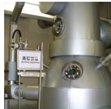
Distillation recovery equipment for waste isopropyl alcohol
