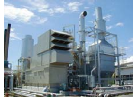
Cogeneration system (Shizuoka Plant)
