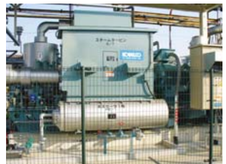
Steam turbine compressor (Shizuoka Plant)
