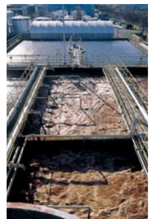
Active sludge treatment equipment (Shizuoka Plant)
