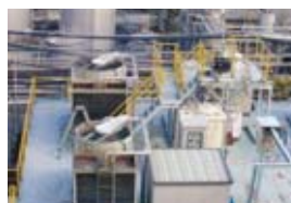
Water recirculation equipment (Amagasaki Plant)
