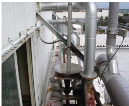
Measures to prevent resin release from the reaction vessel (Shizuoka Plant)
