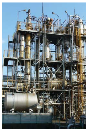
High-precision phenol recovery equipment (Shizuoka Plant)
