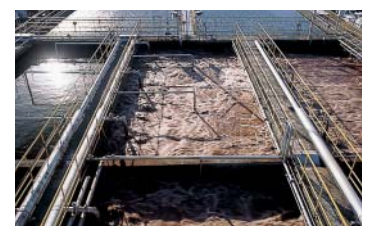
Active sludge treatment equipment (Shizuoka Plant)
