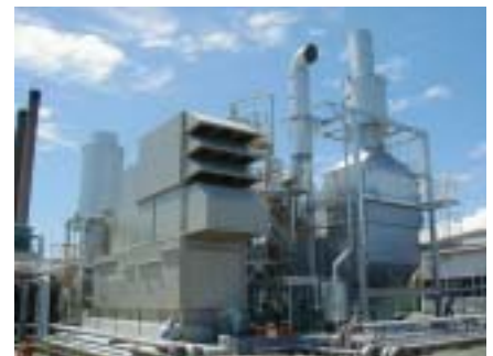
Cogeneration system (Shizuoka Plant)
