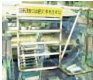
Installation of safety barrier to prevent pinches and entanglements in a roller (Shizuoka Plant)
