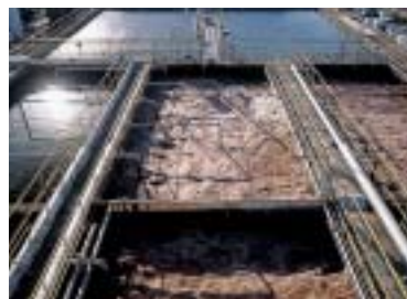
Active sludge treatment facility (Shizuoka Plant)
