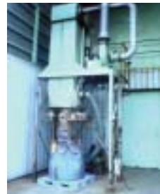
Improvement of work environment for dust collection in flexible container cleaning (Akita Sumitomo Bakelite Co., Ltd.)
