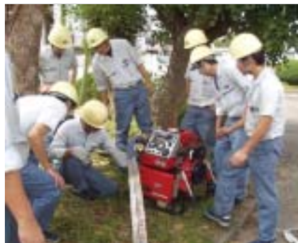
Portable power pump drill (Tsu Plant)
