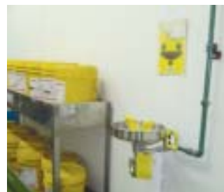
Emergency shower and eye shower (SB Flex Philippines, Inc.)
