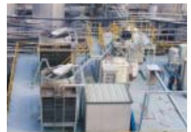
Water recirculation equipment (Amagasaki Plant)
