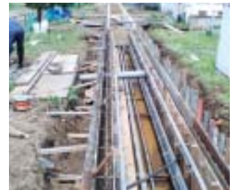
U-shaped construction of trench for outdoor buried pipelines (Akita Sumitomo Bakelite Co., Ltd.)
