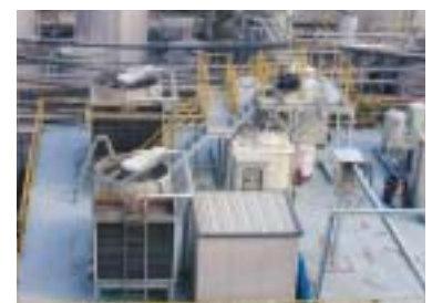
Water recirculation equipment (Amagasaki Plant)
