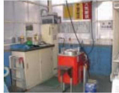
Equipment for distilling and recovering acetone
