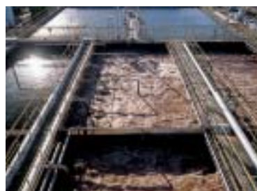
Activated sludge treatment equipment (Shizuoka Plant)
