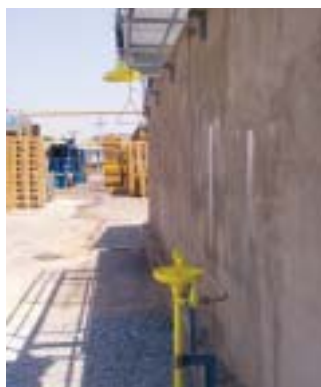
Shower and eye-rinsing unit installed as safety equipment (Fers Resins, S.A.)
