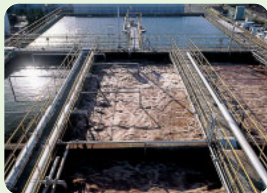
Activated sludge process equipment
