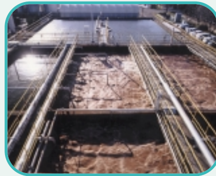
Activated sludge processing unit
