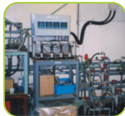
Wastewater monitoring apparatus
